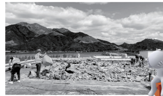
Difficult Renovation, Long Period, High Cost
